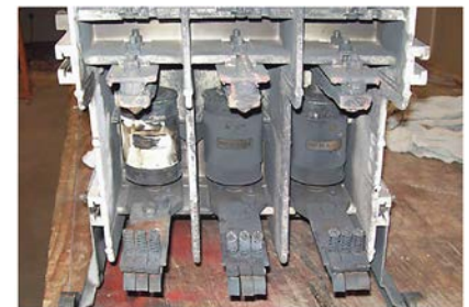
Above is a switchgear contactor after a 5 kV arc-flash event during which traditional overcurrent protection was applied. The damage required replacement of the contactor, fuse clips, copper bus, cable, control wiring, disconnect mechanism, and hardware.
