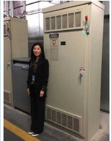
VFD Powering a 350 HP motor
