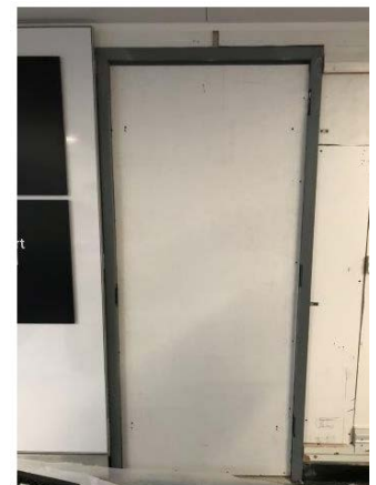
Corridor Level – New Maintenance Access Doors
